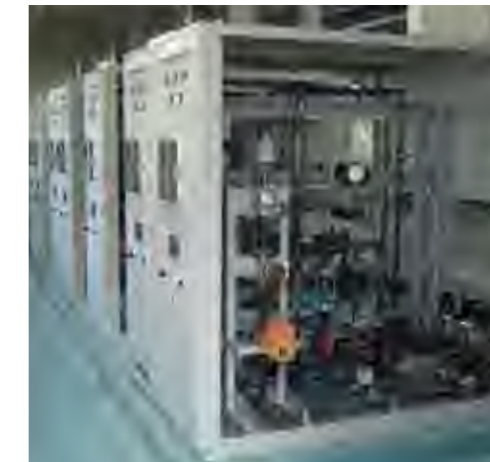
MF-type chemical injection system
