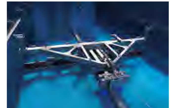
Single wire-type clarifier
