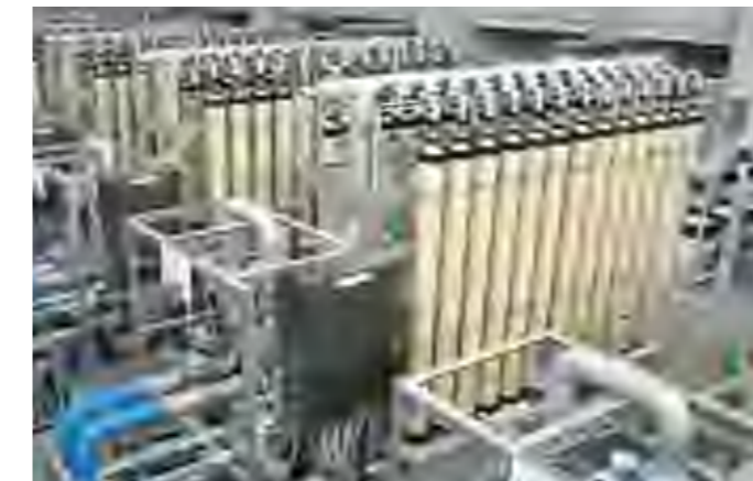
Membrane treatment system
