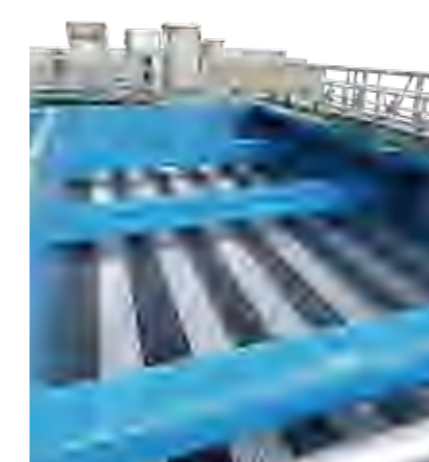
Inclined tube settler
